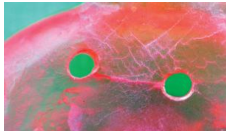
Figure: 2 crackling and cracks in the surface
