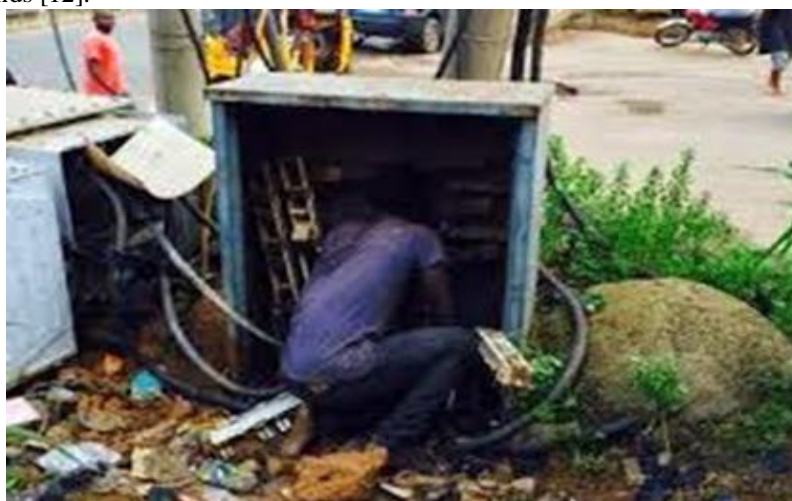
Fig. 4: A Vandal electrocuted in a distribution transformer (Source: Usman, 2014)
