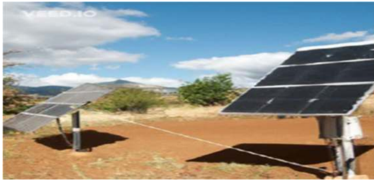
Fig. 1. Showcasing off-grid and grid-tie PV arrays.
